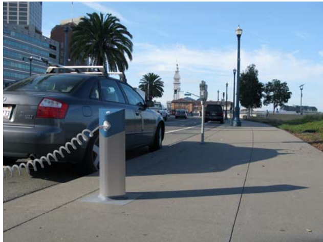
Figure 3 Better Place charging point in California (USA)
